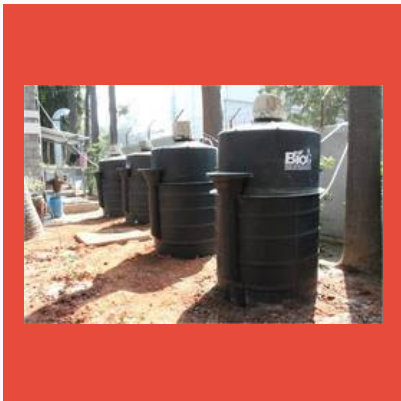
Biogas Plant (Domestic)
